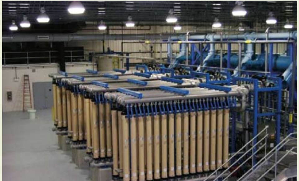
Figure 2. Membrane Units installed post-clarifier at a WTP
